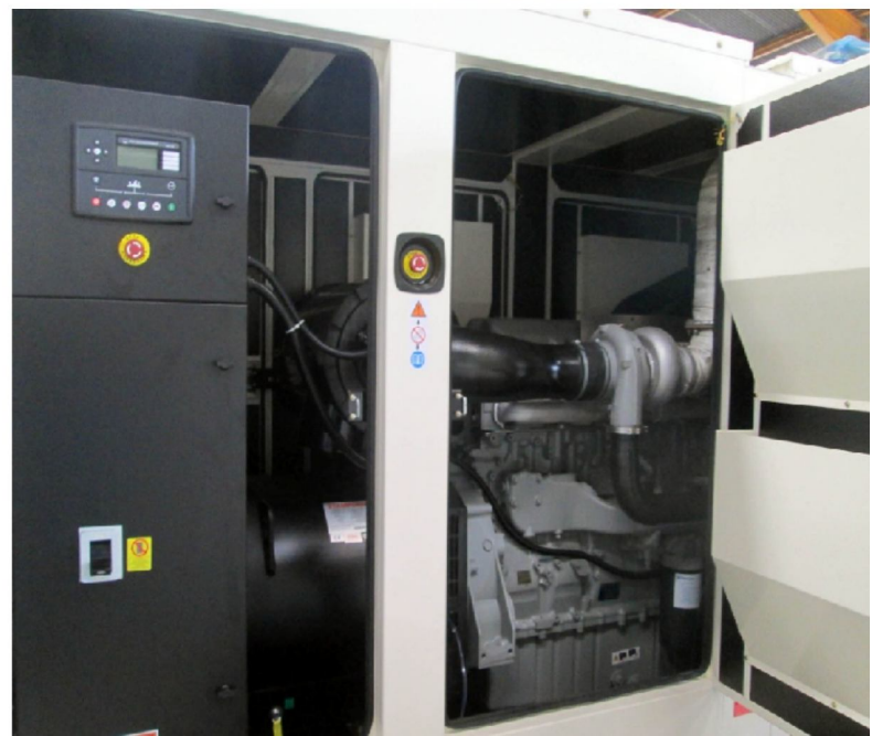
Perkins 2506C-E15TAG2 – 500 kVA Project Luwak White Coffe
